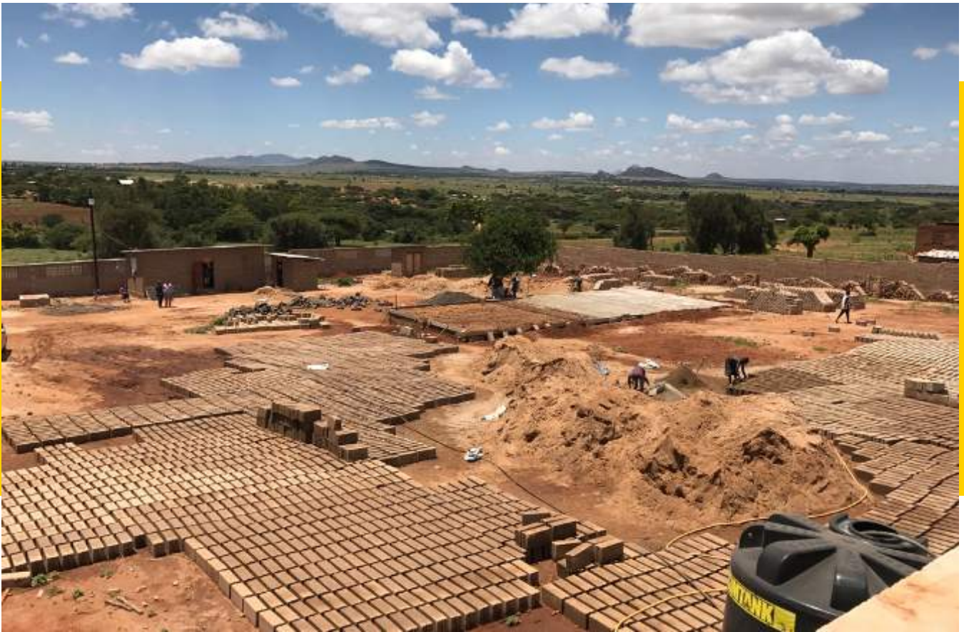
The land at the beginning of the work and surrounded by the fence, March 2018
